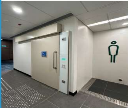
NABCO Automatic Sliding door Immigration HQ Disable Toilet
